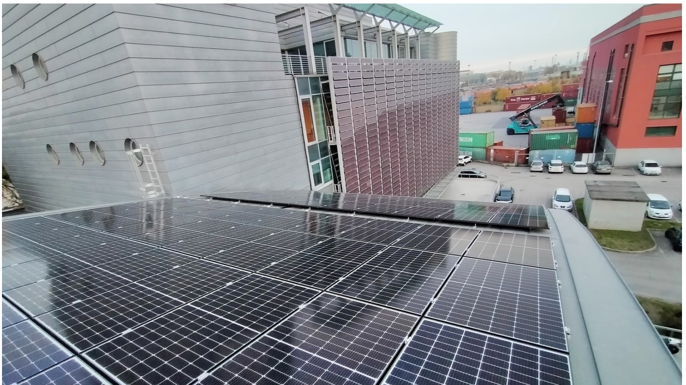
A 70 kWp solar installation from ERRECI in the port of Marghera near Venice.
